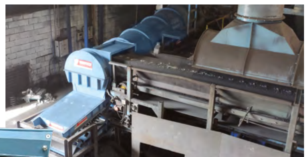
Mold dump conveyor
